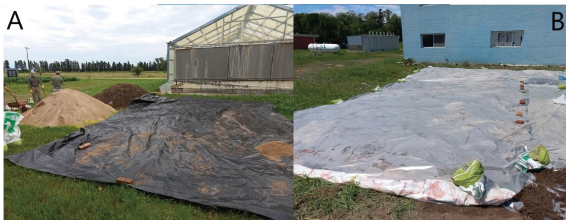
Figure 2. Assembly of the solarization system. A. Section of silo bag placed with its black side up. B. Upper covering of the solarized with polyethylene crystal
